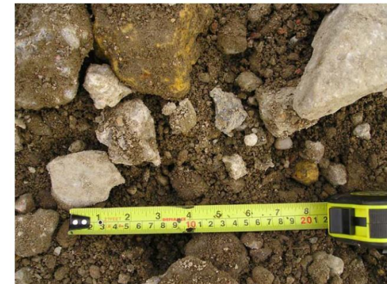
Photo 2 Platform material that has been degraded in use
